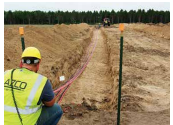
The DC feeders being laid in this trench will route electricity produced by solar panels.
