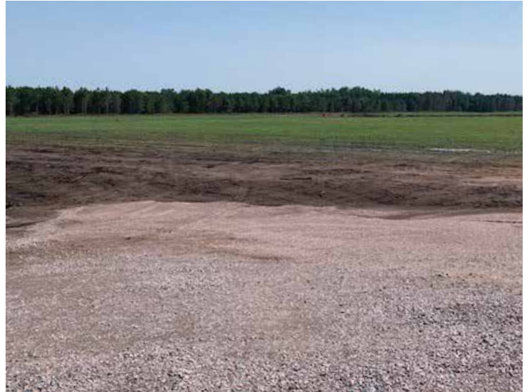
From the base of operations where the office trailers are located and the equipment is parked, this view to the northeast shows the area that is furthest along with vegetation growth already making strong progress.
