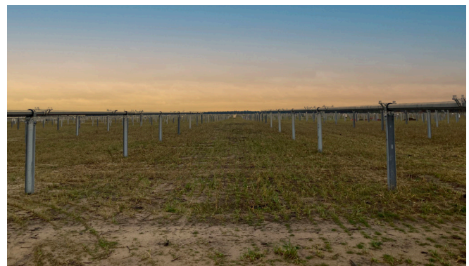
Piles and racking fully installed and await solar panels (Wood County Solar Project, Wood County, WI).
