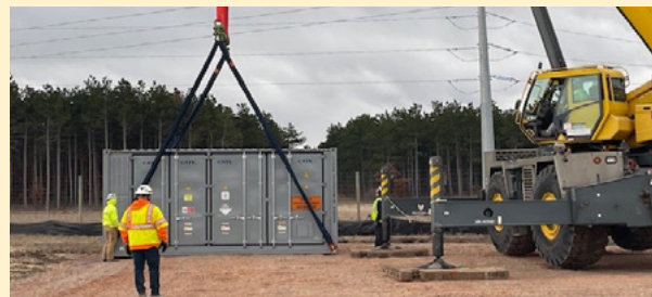
Battery energy storage units arrive on-site adjacent to the Wood County Solar Project.
